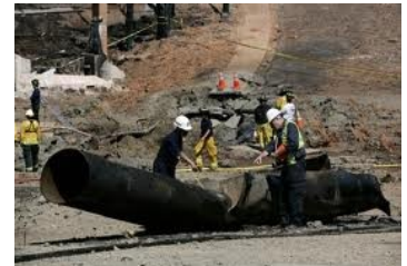
Investigations revealed that portions of the San Bruno pipeline contained welded seams despite PG&E records showing the entire line to be seamless.
